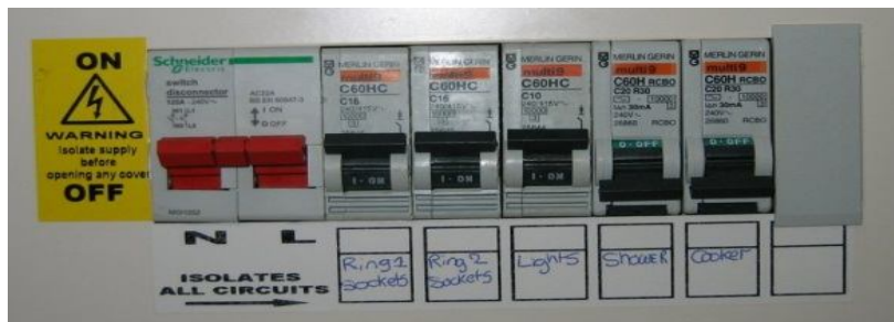
Figure 2: A switch board which shows several circuit breakers already installed.
